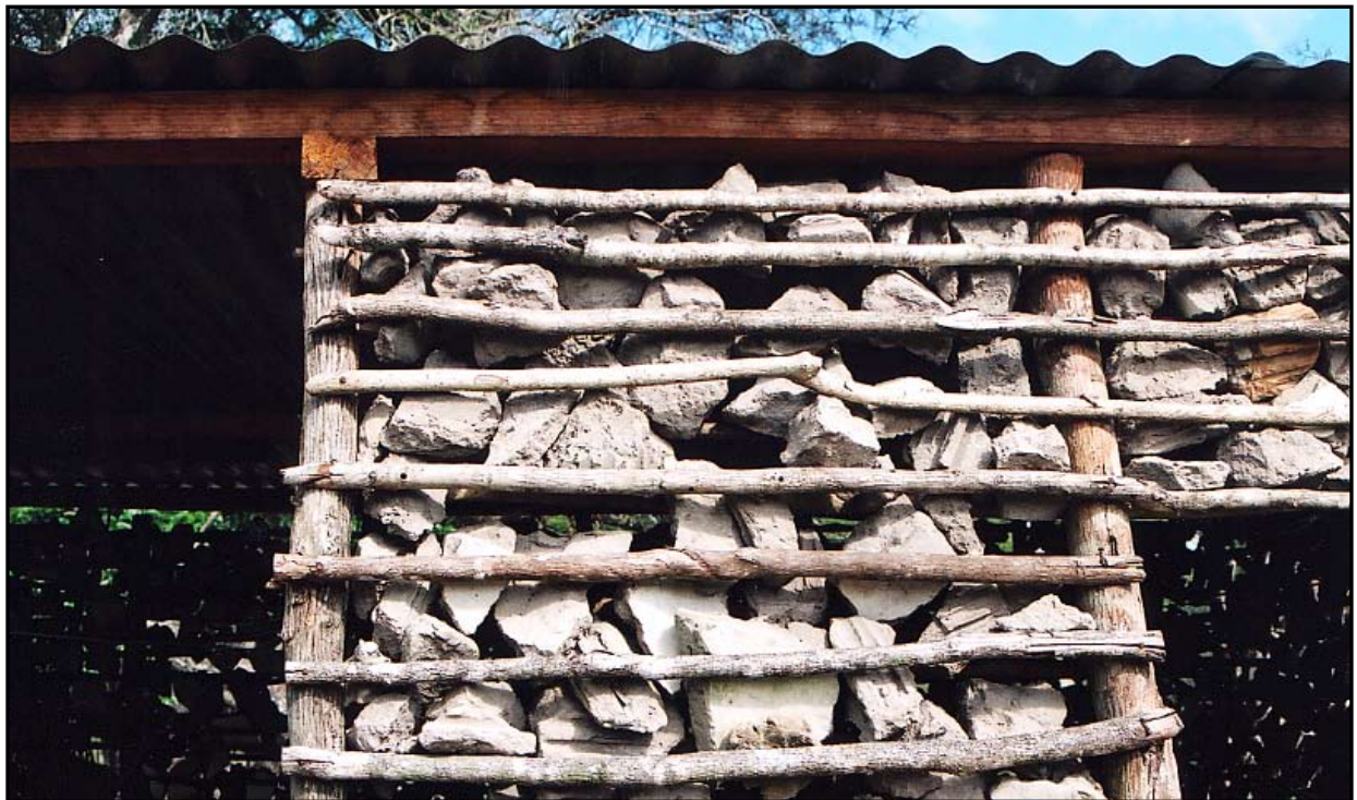
Figure 5. An example of a wood and stone wall, with the space between the horizontal wooden laths filled with old concrete rubble. Community of Manqakulane, Maputaland, KwaZulu-Natal province, South Africa, as established by a survey in 2002.
